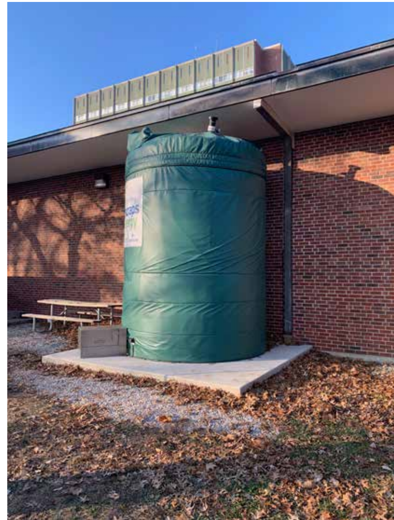
Ground dining hall food waste is emptied into the Grind2Energy holding tank (pictured). The slurry is transported to the Urbana-Champaign Sanitary District's anaerobic digester for electricity production.
