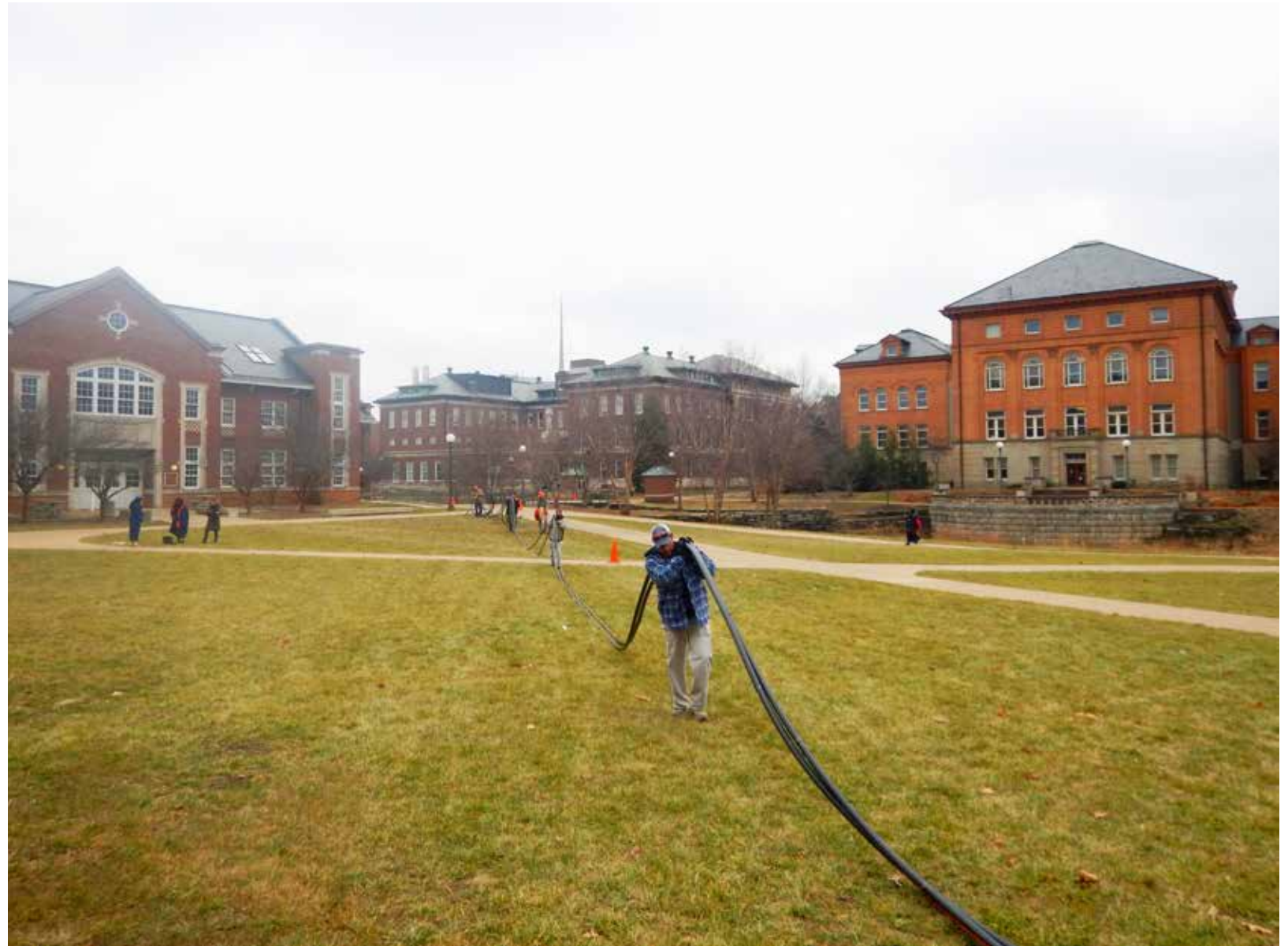
Geothermal loop and fiber optic cable installation on the Bardeen Quad, December 2018.
