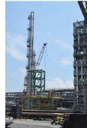
Linde 1.5 MWe Capture Plant at National Carbon Capture Center
